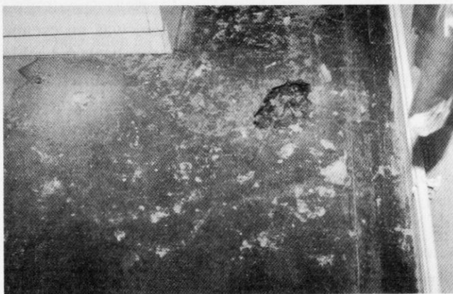
First impressions. Rubble suspended on mineral felt membrane in Room 16 at Denton House on 10 December 1992. Photo by Peter Bailey
